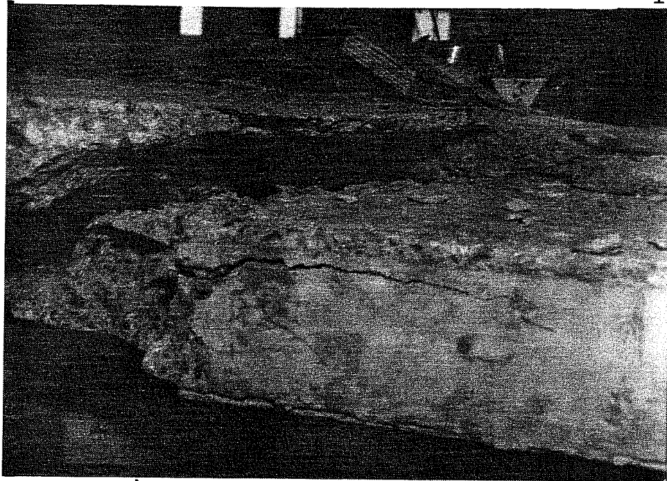
a).- Top flange condition at failure
